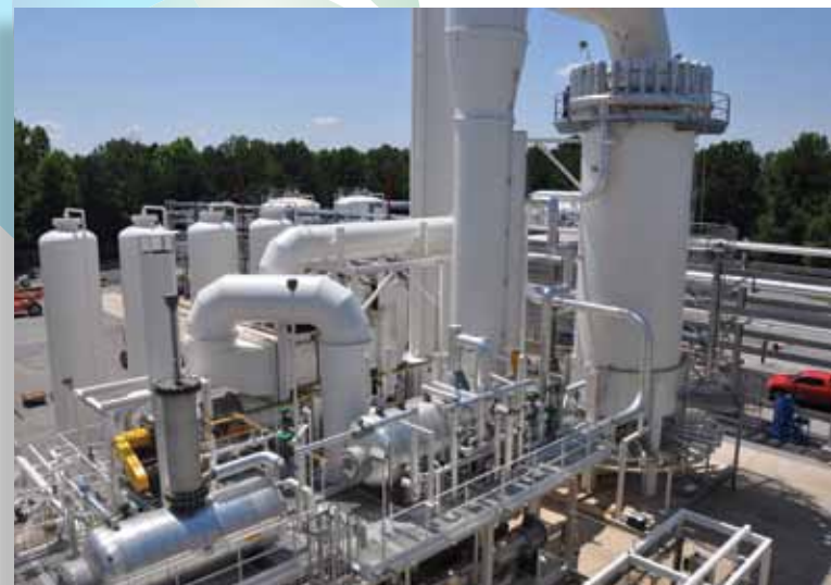
MATHESON Hydrogen Plant at a Biofuels Refinery
