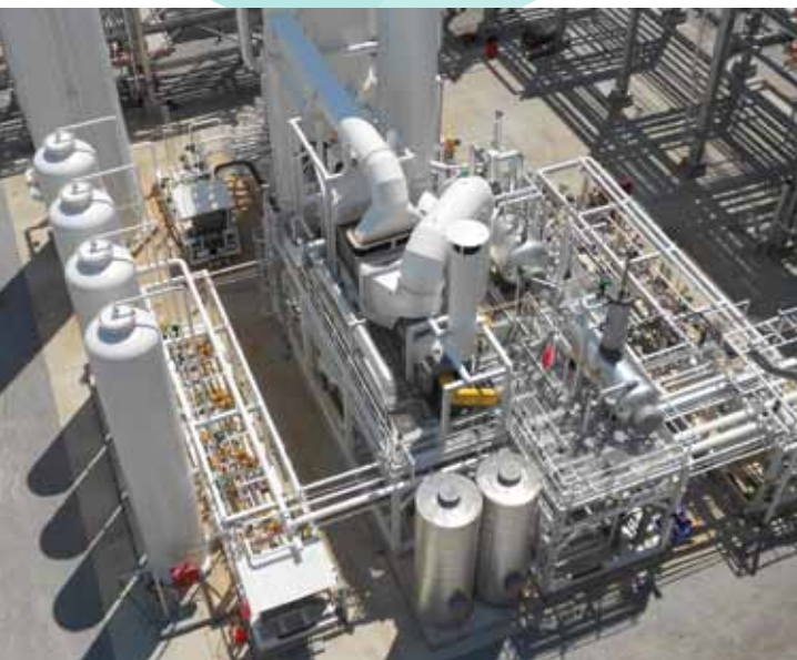
MATHESON Hydrogen Plant at Refinery Customer
