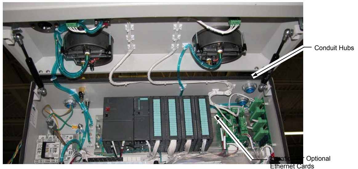
Figure 6. Typical PLC in Controller Enclosure
