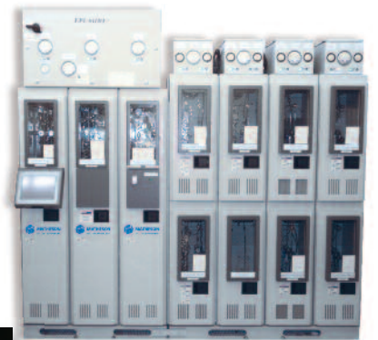
Point of use purification to assure process consistency.
