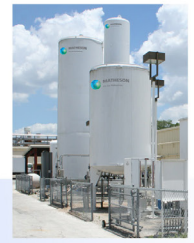
Onsite Plants and Pipeline
