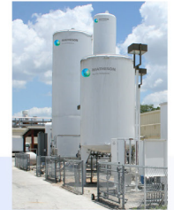
Onsite Plants and Pipeline
